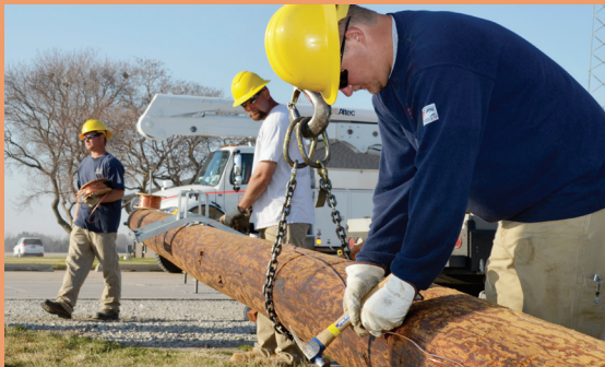
Line Technicians (from left) Jim Baumert, Clint Williams and Eric Brabec install a three-phase service. May, 2015
