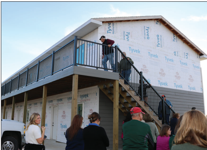
The 14-unit complex features seven units on top, and seven on the bottom. They are two bedrooms and one-bath units. Construction is still ongoing with hopes of having occupants early next year.
